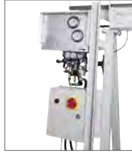
Detail of the control panel.
