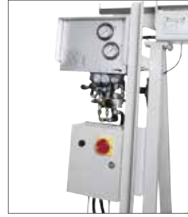
Detail of the control panel.
